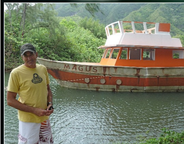
"This is the Magus midway through construction. While a real boat was used in the pilot, it was impractical for many reasons. So I devised a plan to make a floating set that draws a mere eight inches."
